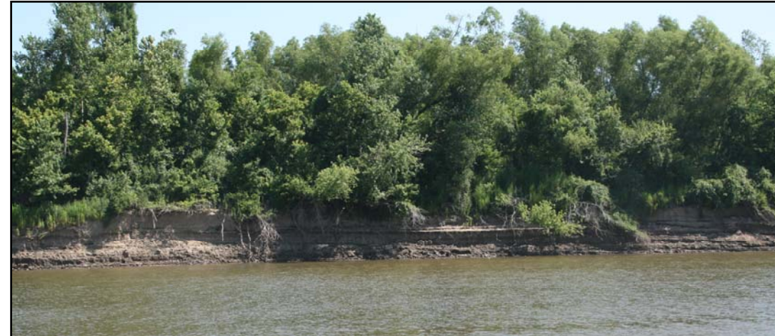
Bankline erosion on the LDB of Salt Lake Chute
